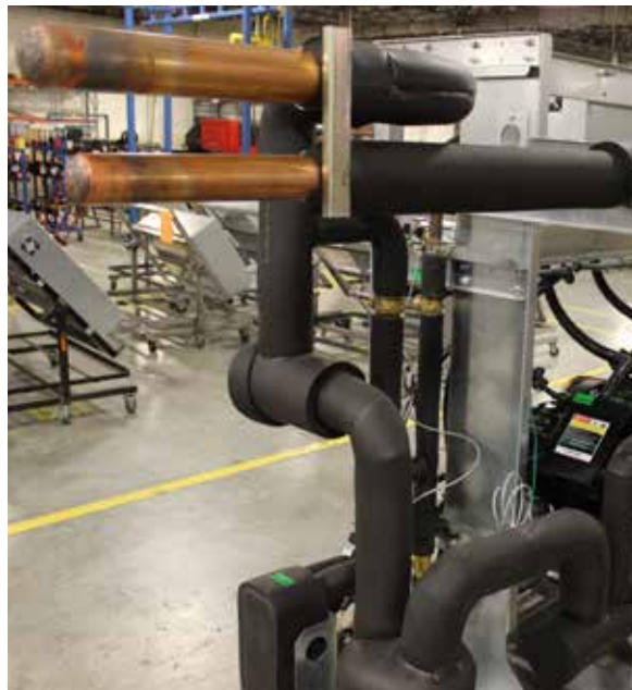
Figure 1-18. Example of the single pair of in a loop configuration leaving/returning to the rack (before being hooked up)
