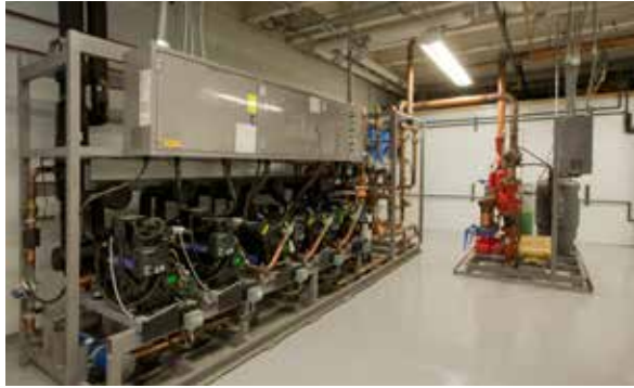
Figure 3-7. Rack Mounted on Floor
