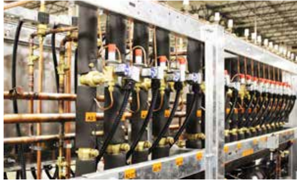
Figure 1-16. Example of a Rack for a Circuit System
