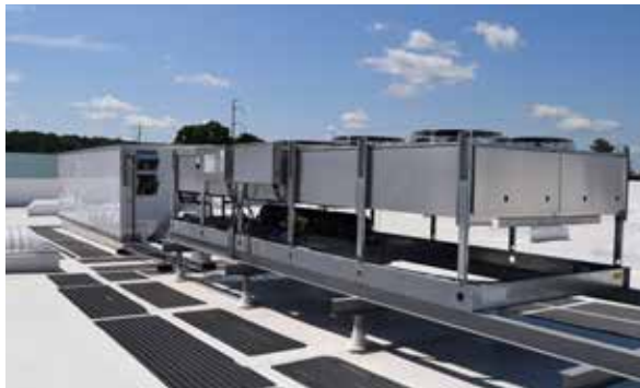
Figure 3-8. Equipment Mounted on roof
